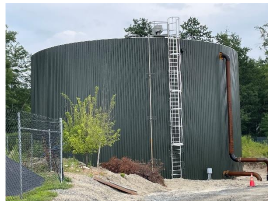
60,000 gallon cold water storage tank at Little Leaf Farms – July 2023
