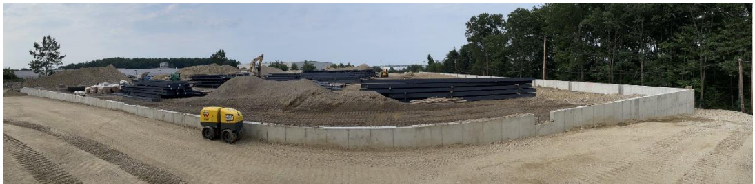
View of the foundation walls for the new building at 35 Saratoga – August 2023
