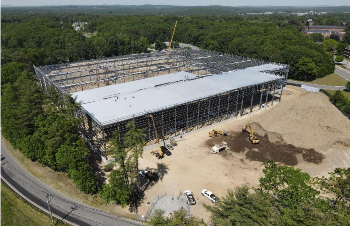
Top: aerial view of the front of 11 Grant Road under construction. Bottom photo is the rear – June 2024. Photos courtesy of Mack Devens, LLC.
