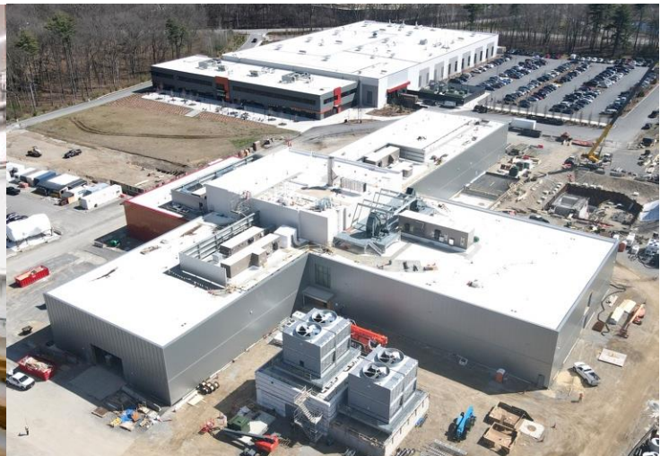
Rear of CFS SPARC facility – June 2024. Photos courtesy of CFS.
