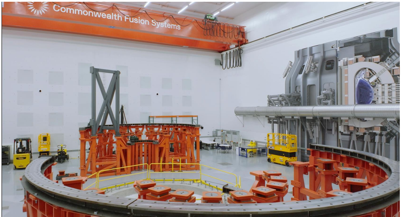
*Interior of SPARC – (“Tokamak Hall”) under construction – 2024. Photo courtesy of Commonwealth Fusion Systems
