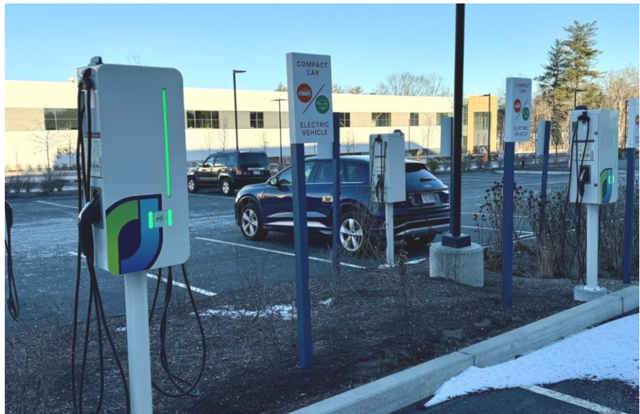
New electric vehicle charging stations at the Pathway Devens Campus developed by King Street Properties. Combining EV charging with compact car parking spaces not only helps reduce carbon emissions from vehicles, it also reduces the amount of pavement which reduces urban heat island impacts and stormwater runoff. Adjacent biofiltration landscape islands also help manage stormwater runoff and integrate more natural elements into the urban landscape.
