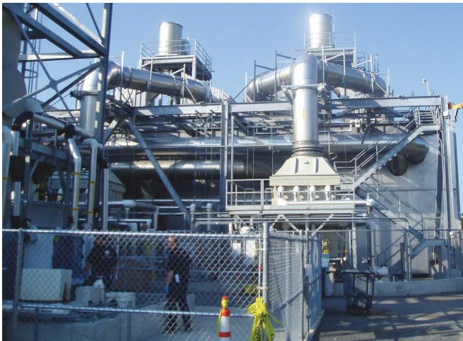
Before: 112 Barnum Road Pollution Abatement Equipment (above—July 2009).
