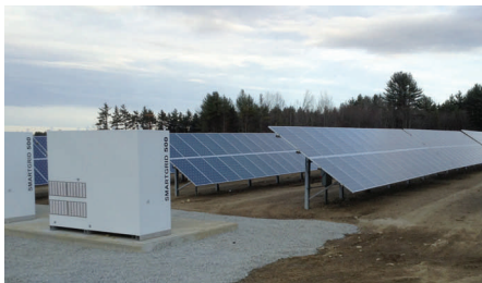
Ground-mounted solar photovoltaic panels and smartgrid power inverter boxes in the EBZ.
