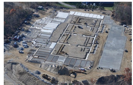
A birds-eye view of the New England Studios sound stages as workers prepare the concrete walls to be hoisted into place..
