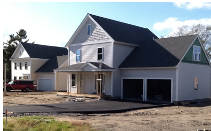
Transformations, Inc. finishes Construction on two of the eight single family energy efficient homes.
