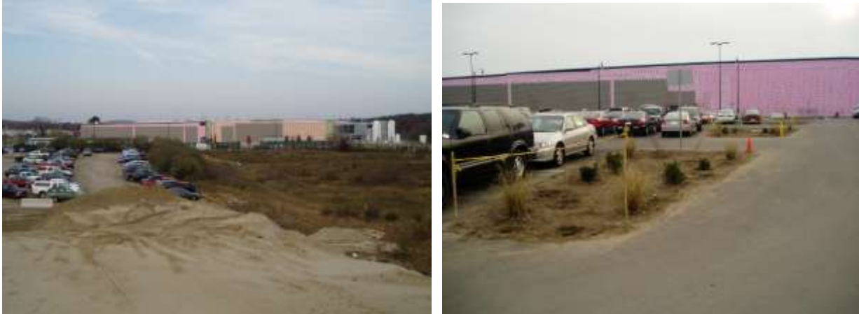
Looking northeast from Barnum Road (west side of bldg. and Utility Yard) Planted rain gardens in parking lot. Building siding being installed
